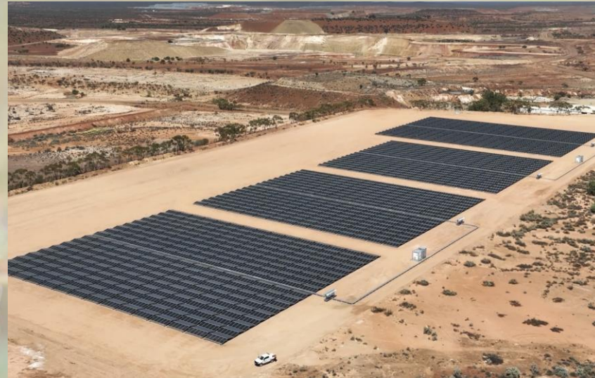
Solar farm at Mt Magnet
