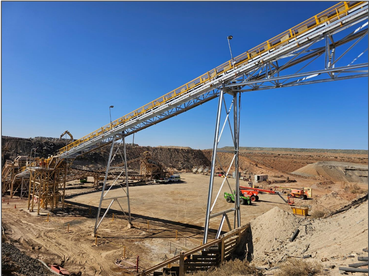
Figure 5: New sections of CV01 at Mt Magnet processing plant
