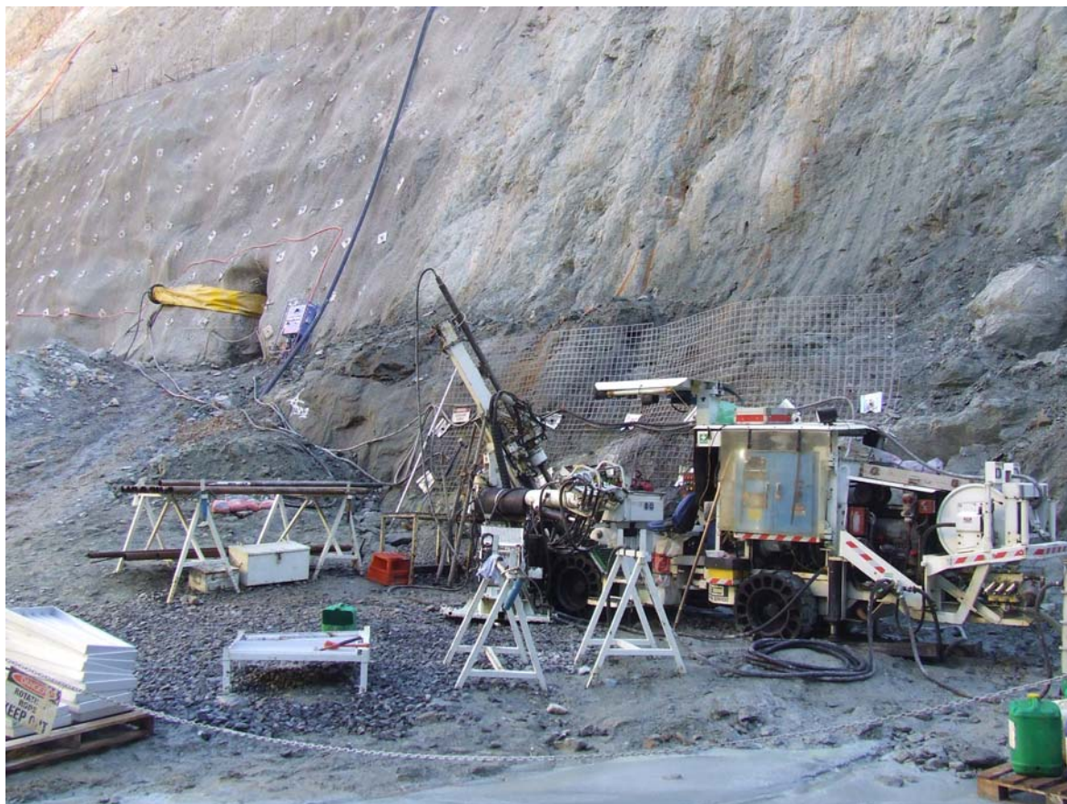
Swick Diamond Drill Rig in Wattle Dam Pit with Escapeway Portal in background
